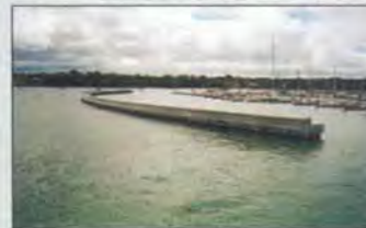
Sandringham Yacht Club, Victoria, Australia. 3,000 sqm. Radcon #7 applied to this pre-cast wave barrier for concrete protection.
