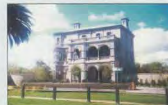
Heritage Building, Melbourne, Australia. This single skinned rendered building had leaked through the facade for many years. After several coats of paint were removed Radcon #7 was applied to stop all leakage.
