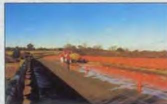
Perth Bridge, Tasmania, Australia. 2,600 sqm. Radcon #7 applied directly onto exposed structural concrete that was eroding from traffic & freeze/thaw damage.
