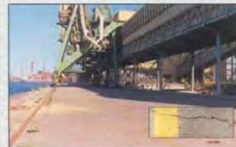
Grain Berth, Port Kembla, Wollongong, Australia. Radcon #7 alone, was used to seal these leaking cracks up to 2,00mm.
